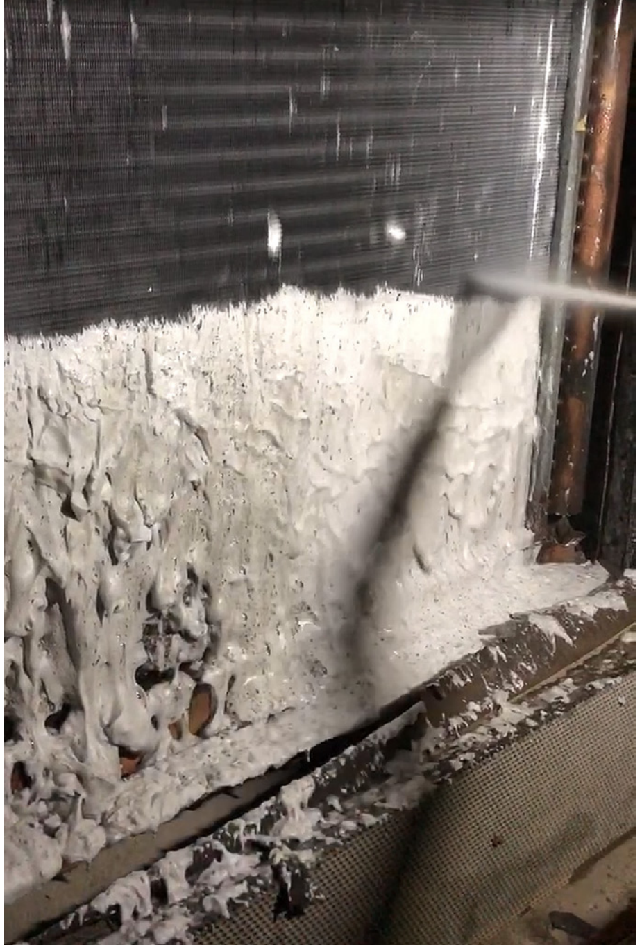
Coil washing and disinfection to maintain its cleanness and performance
